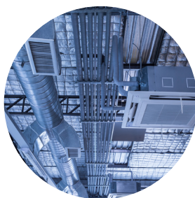
HVAC and ventilation systems
